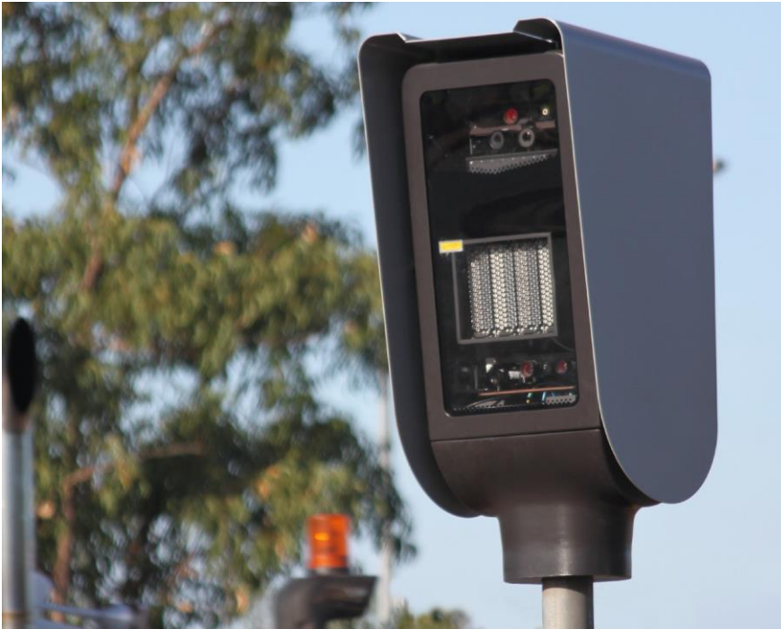
Redflex bus enforcement system mounted on existing infrastructure.
