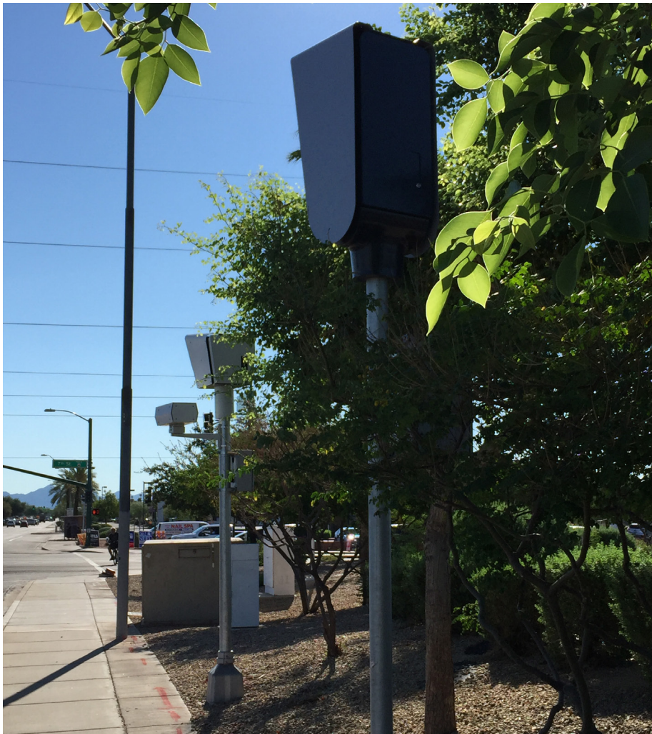
Redflex's test site in Phoenix, AZ with our new Halo technology.
